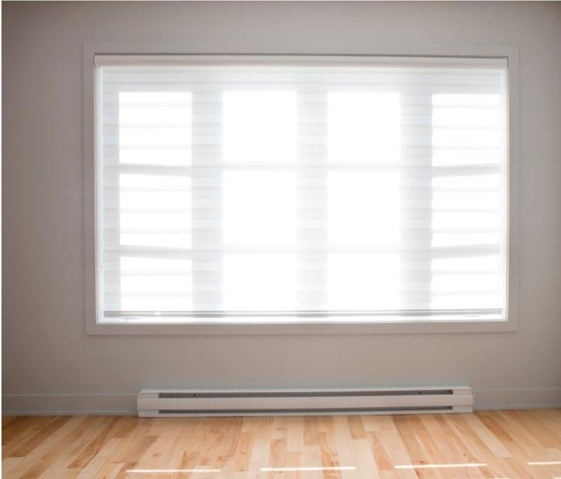
Figure 1 - Electric baseboard unit under widow
